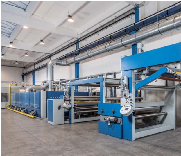
Monforts ATC | Germany
